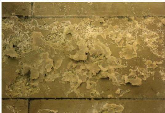
Fig. I-5. Efflorescence, Crypt of the Cathedral of Cádiz, Spain (Limestone) (Vázquez et al., 2011).
