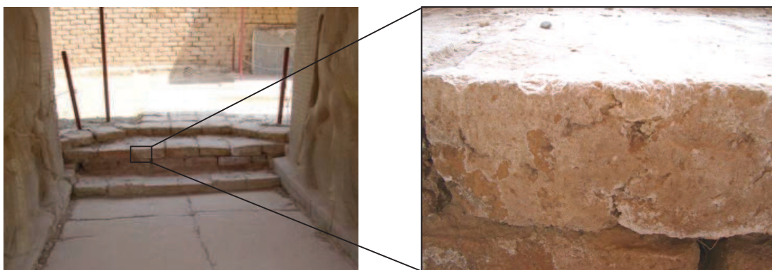
Fig. I-7. Granular disintegration by salt weathering, Al-Nimrud monument, Iraq (Limestone).
