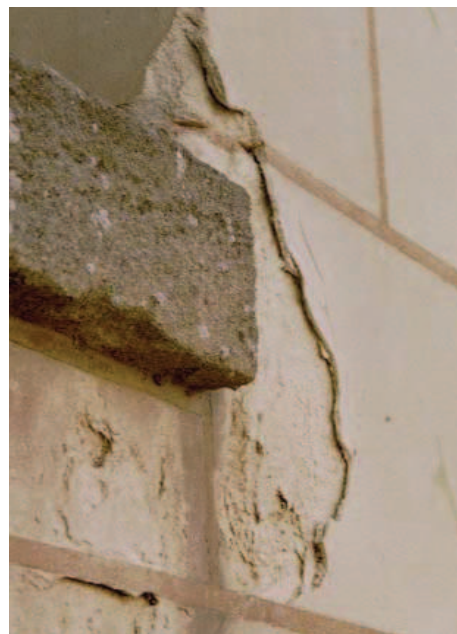
Fig. I-16. Stone degradation by contour scaling, Castle of Chambord, France (tuffeau limestone) (Beck, 2006).
