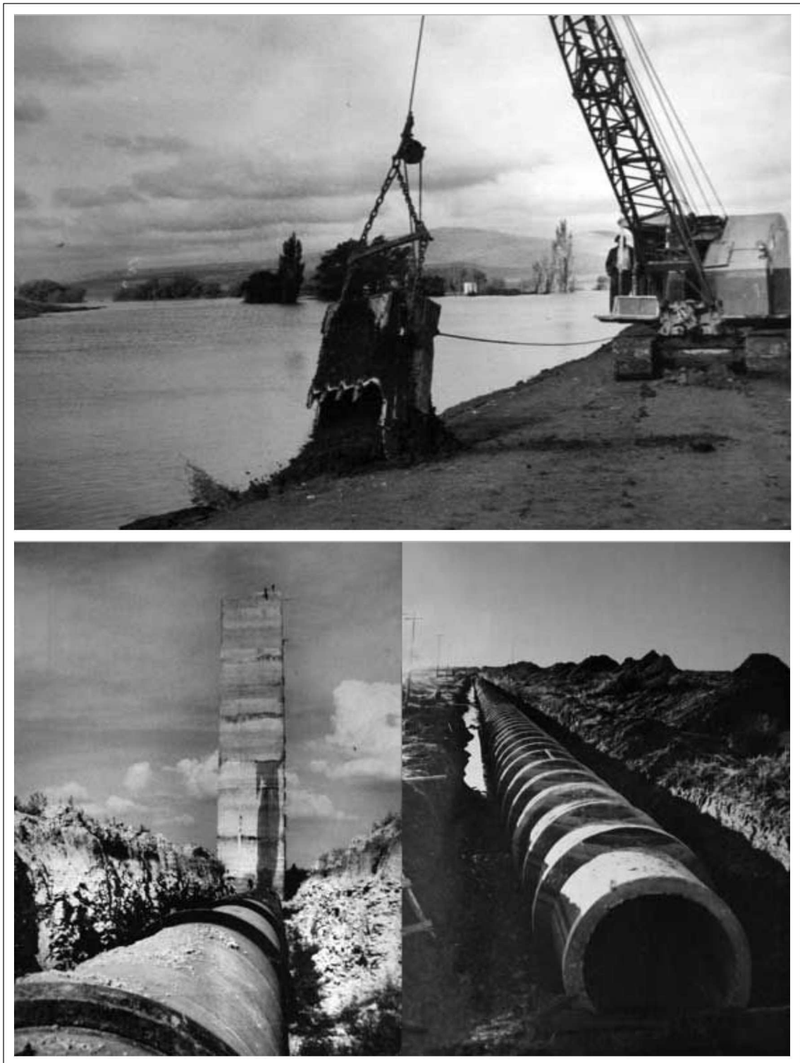
Figure 5.25: Operations for dam construction by early 1970's. Source: La Nueva Provincia ( http://www.lanueva.com/multimedia/nota/3855858f4a/173/18136.html ).
