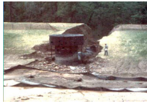
Erosion interne, Barrage Loveton-1989 (ASDSO, 2009)
