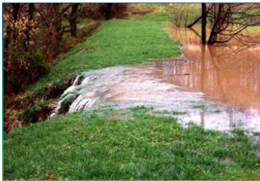
Erosion externe (ASDSO, 2009)
