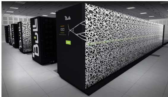
(a) Tera 100 Supercomputer
