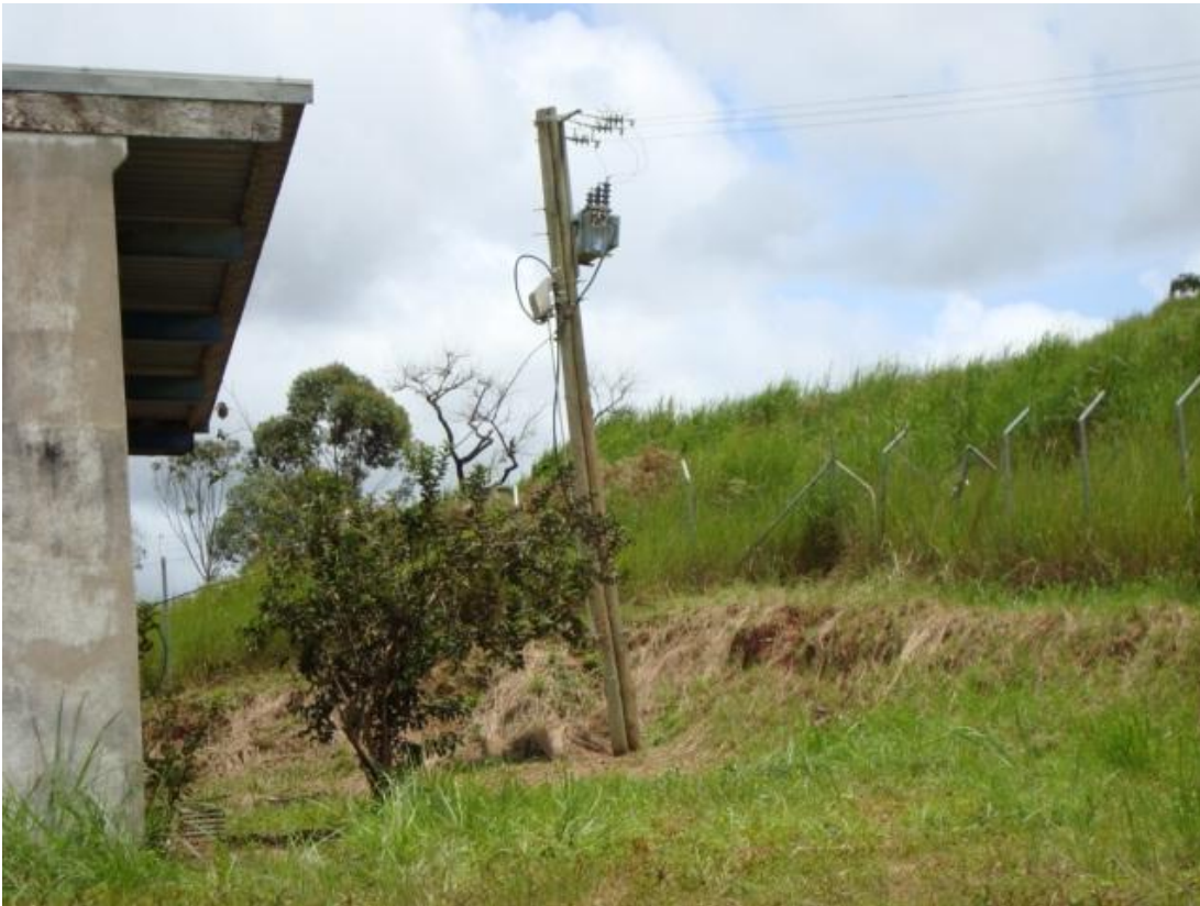
Plate 4: Newly repaired transformer just before our visit in August 2011, Ngefor G.S., 2011
