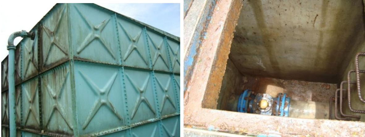
Plate 12: Old Water tank constructed by the Germans with the meter calculating the total water supplied out of function. It is thus impossible to know the exact water supplied in Bali
