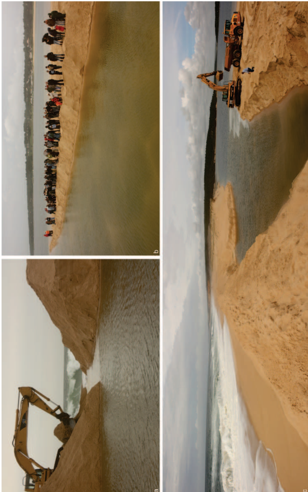
Figure 3.21: Opening of the Albufeira Lagoon inlet on 28 March 2013. a) Discharge of the lagoon water into the ocean; b) The local population attending the traditional "abertura da barra"; c) panoramic view of the channel before opening.
