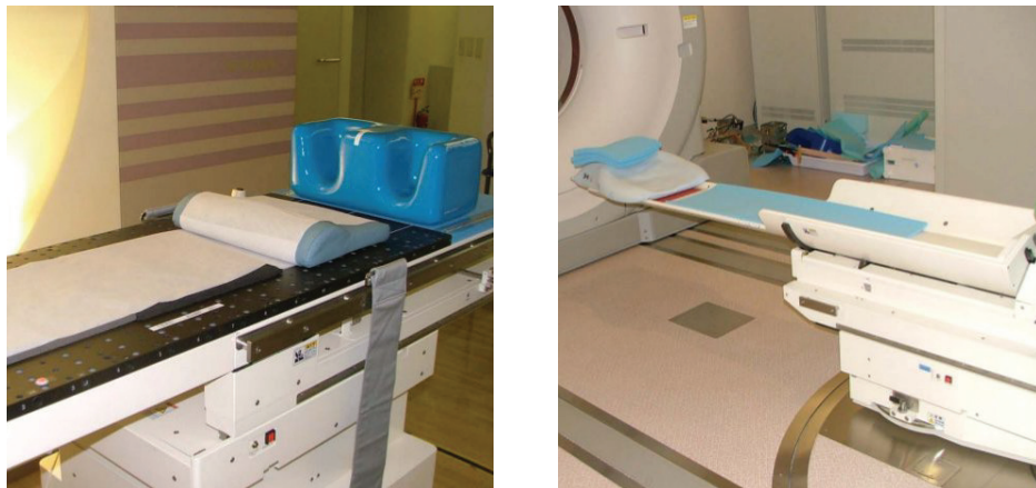
Figure 1. a) Flat table top (indexing system and standardized knee and feet supports visible) at HIMBC facility; b) Rotating patient cradle (installed in CT room) at GHMC facility.
