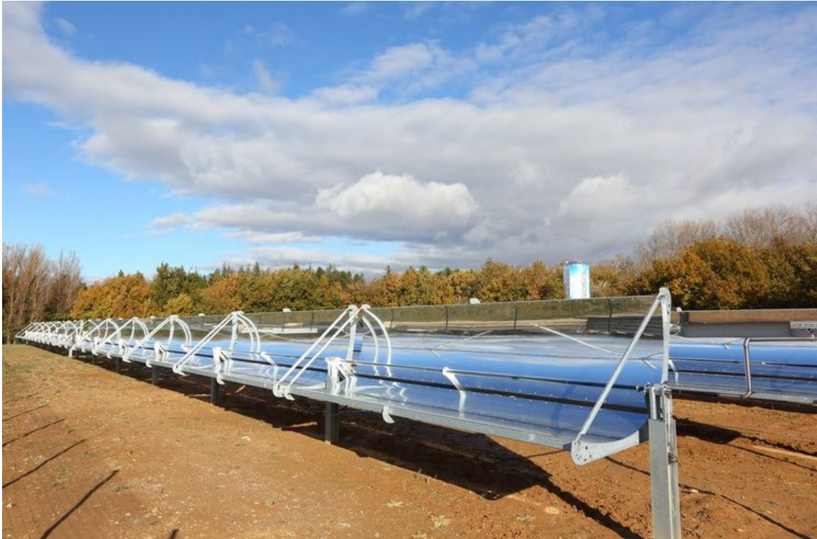
Figure 2.4: Parabolic trough mirrors constituting the solar collector field of the ORC based power generation system
