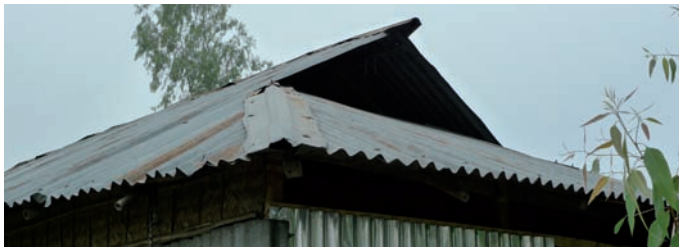
4 slopes roof: ridge piece with pointed shape to break the wind flow
