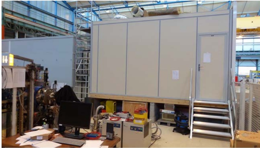
Figure 13.7: The laser hut built in the GBAR zone (the positron trap can be seen on the left); picture taken during the installation of the air conditioning unit.
