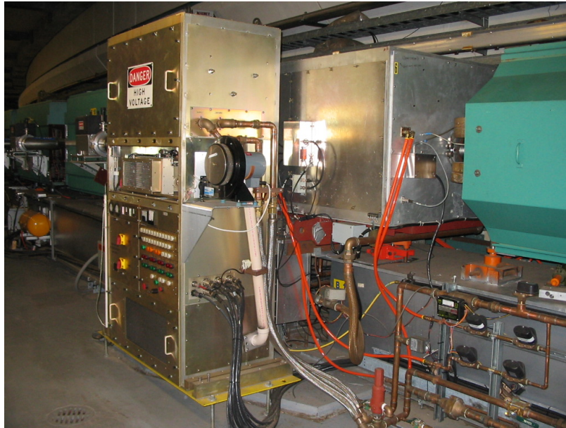
Figure 2.7 Picture of the RF station located in the straight section B10 and seen from downstream.
