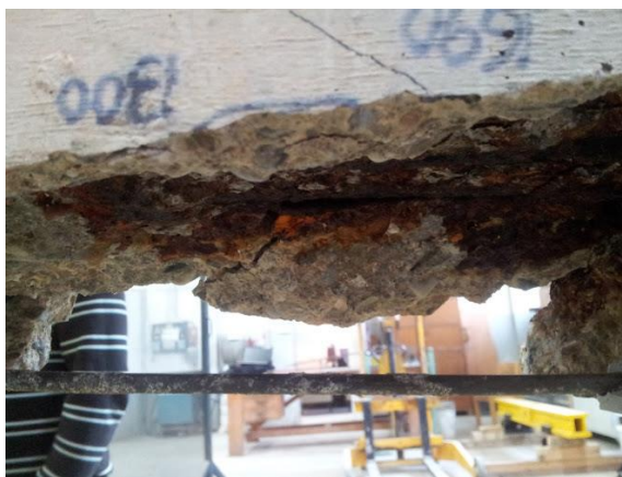
a) A1CL3-R Corroded Beam
