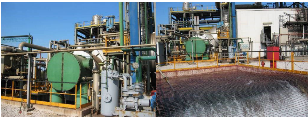
Figure 3-1: Pictures of the Piombino power plant: power plant view (left side) and outlet of seawater in the pool (right side).
