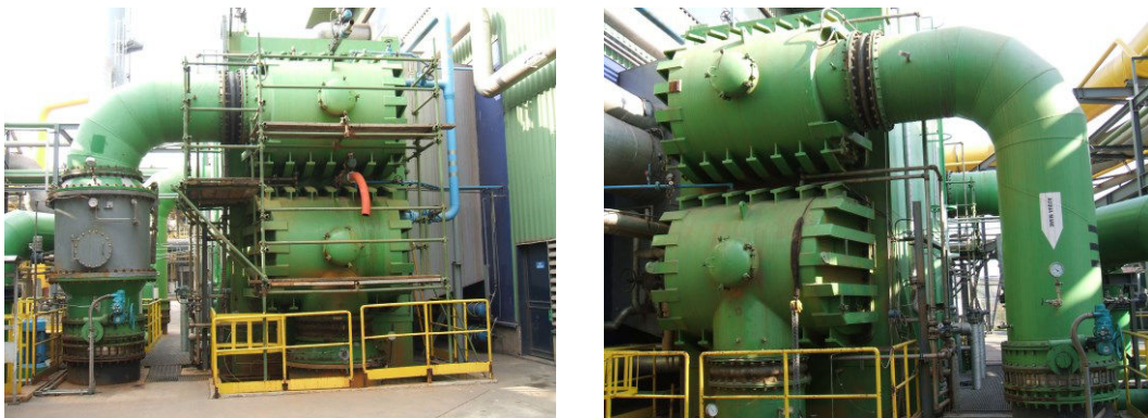
Figure 3-3: Pictures of the heat exchanger at Servola power plant: inlet (left side) and outlet (right side).
