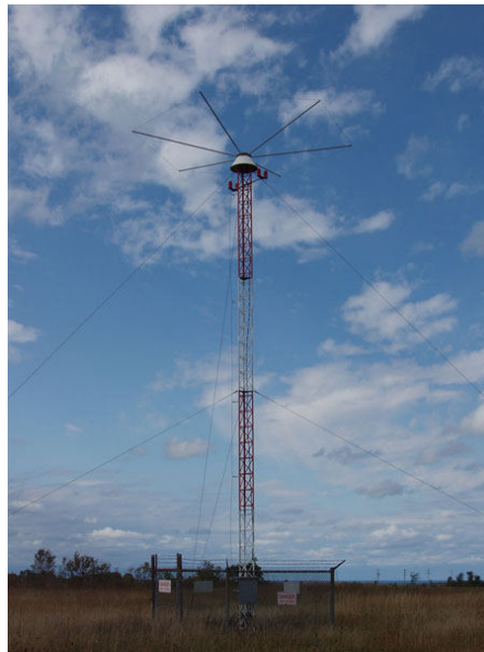
FIGURE B.2: Non-Directional Beacon 6
