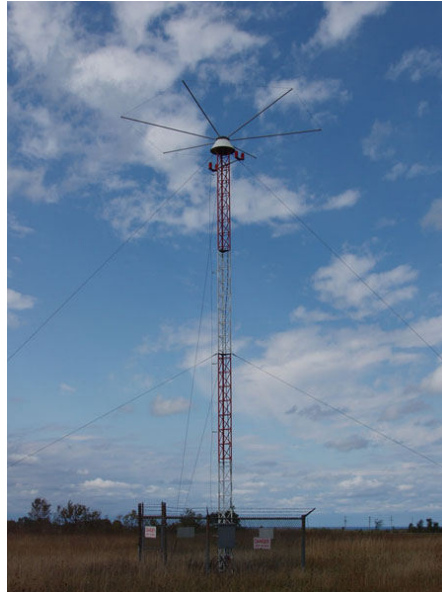
FIGURE B.2: Non-Directional Beacon 6
