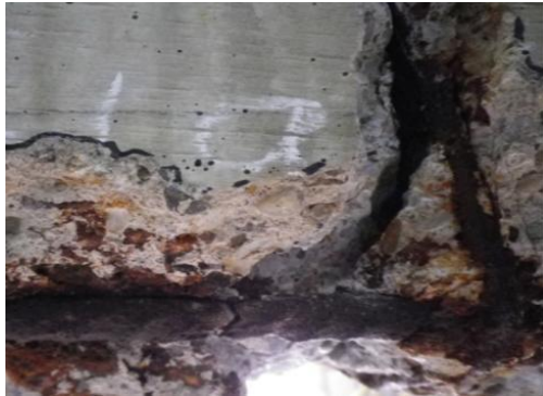
(a) Corroded beam
