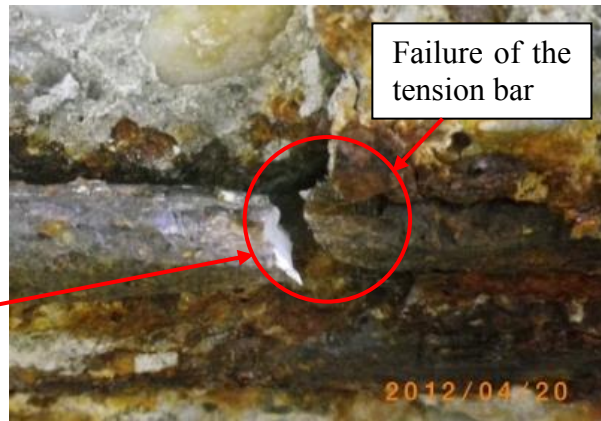
(c) Failure of tension bar of B2C13-2
