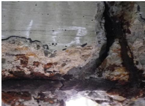
(a) Corroded beam
