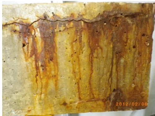
Figure 8-1 Corrosion products in the outside surface of B2Cl3
