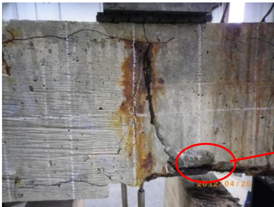
(b) Failure of corroded beam B2C13-2
