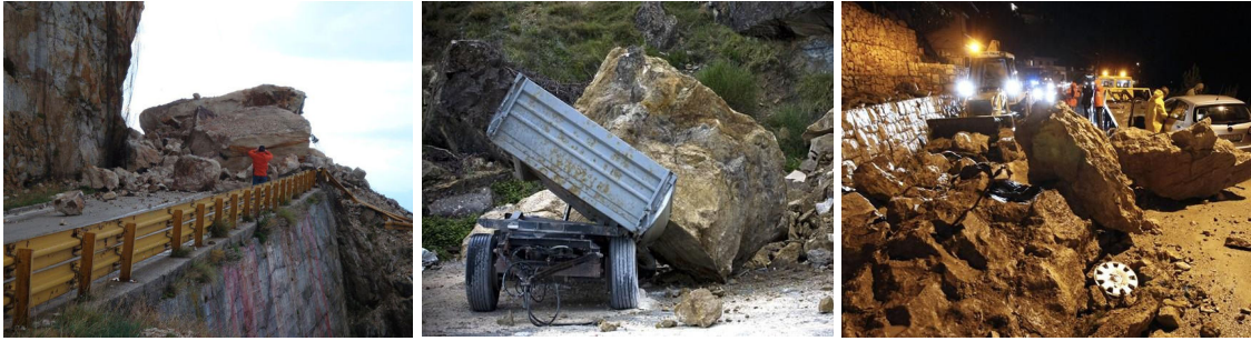
Figure 1.1: Rock falls hitting the coastal roads: Omiš, April 2012.; Omiš, April 2012.; Krilo Jesenice, March 2010.
