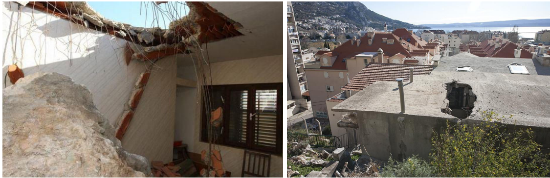
Figure 1.3: Severe damage of houses is caused by rock falls: Omiš, January 2012.
