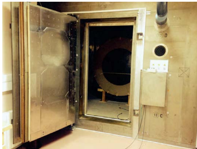
Figure 3.19: Magnetically shielded room at SPEC/CEA Saclay.
