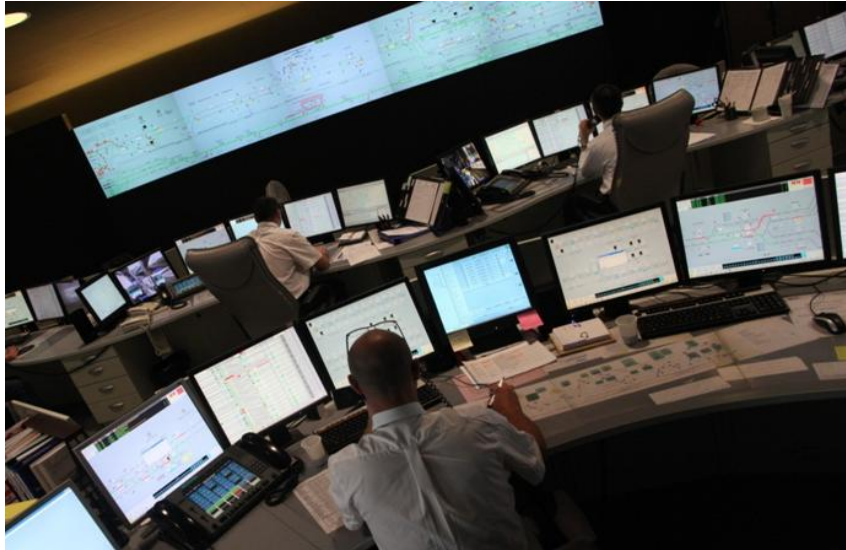
FIGURE I.6 – PCC Ligne 13 - Paris
