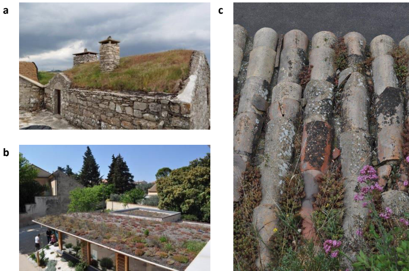
Fig. 1.6 Pictures illustrating installed and natural EGRs in a Mediterranean context. a) Grass roof on an old farmer's house on the Causse Méjean in the Parc National des Cévennes. The colder and humid local climate makes this kind of EGRs possible. b) EGR installed on the Naturoptère in Sérignan-du-Comtat as part of a sustainable building project. This EGR consists mainly of succulent species and is equipped with an irrigation system (sprinklers) that water the EGR every other day during summer at night for two times 15 minutes. The water comes from an underground rainwater harvesting (RWH) well (personal communication). c) Succulent species (mainly Sedum album , S. acre and S. ochroleucum ) and grass species installed spontaneously on the roof of an old Mediterranean building. The plants are able to survive on the spots where water and OM accumulates [Pictures: Carmen Van Mechelen; June 2011].
