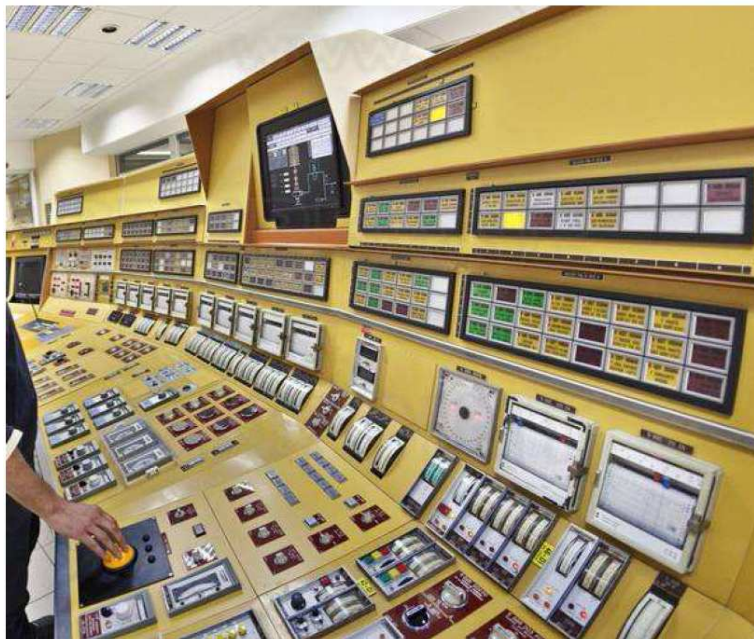
Figure 48: A conventional nuclear power plant control room
