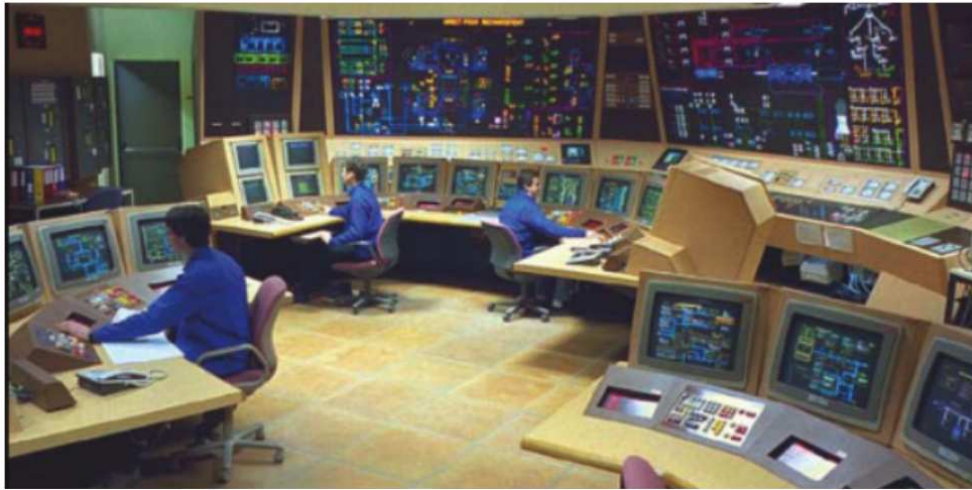
Figure 49: A computerized nuclear power plant control room
