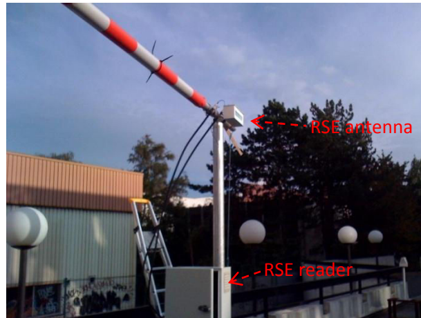
Fig. III-38. RSE antenna mounting detail where the antenna is connected by coaxial cables to the DSRC reader.
