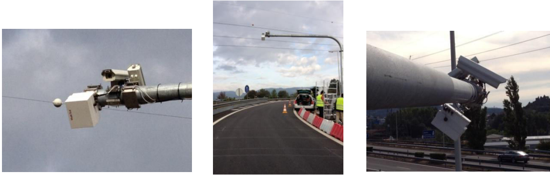
Fig. III-42. Pictures of the Multitoll DSRC system being installed on a Portuguese highway.
