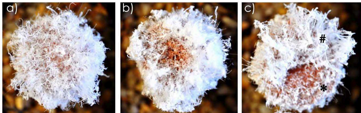
Figure 34. Efflorescence observation on the surface of a GP14.5 geopolymer paste when the surface was dried during the first 24 hours: a) in the open air, b) under protection or c) 50% in the open air (#) and 50% under protection (*).
