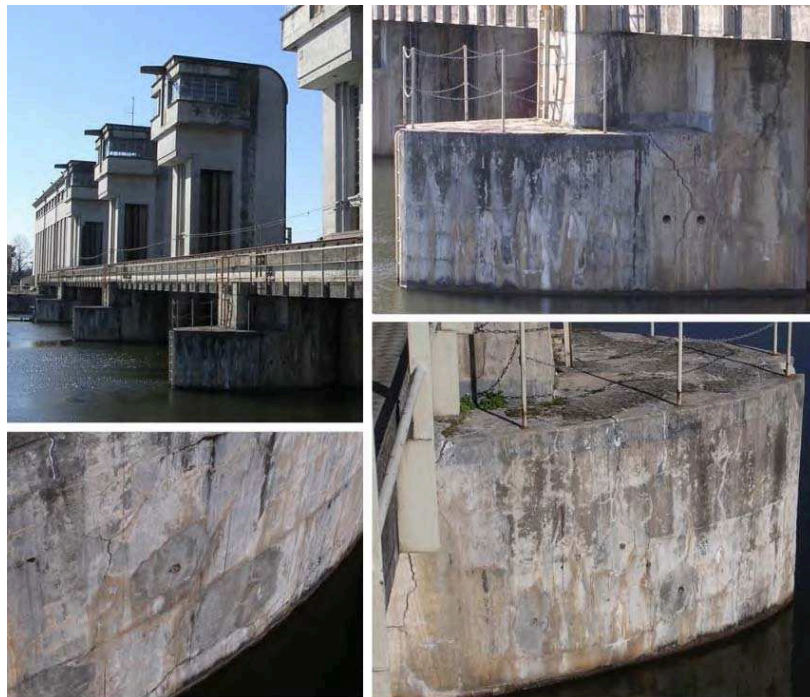
Figure 1. View of an ASR map-cracking pattern in a dam
