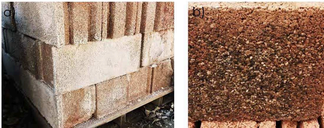
Figure 29. GP MU full unit presenting a) efflorescences and b) surface scaling.
