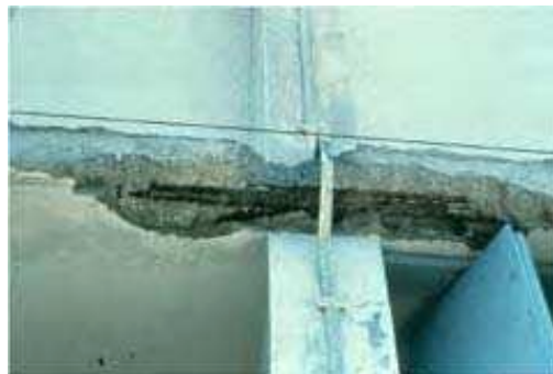
Figure 1. Example of carbonation on a building facade (from http://www.cement.org )
