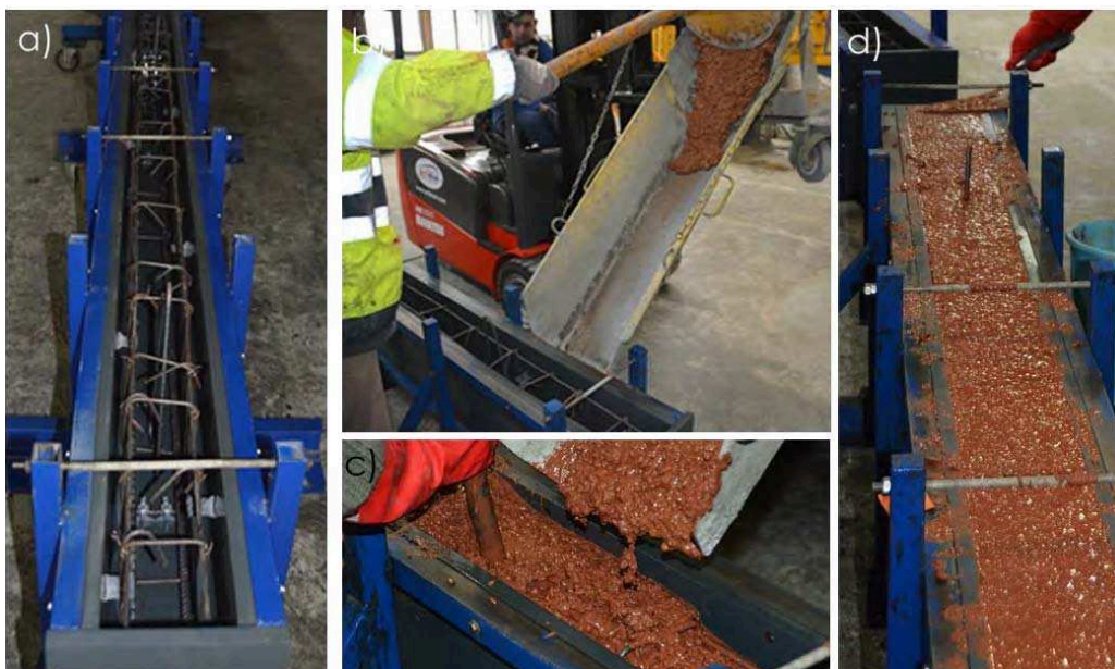
Figure 22. a) Beam mould with the steel reinforcement; b) descent of the fresh concrete by gutter; c) vibration of the fresh geopolymer concrete using a vibrating needle and d) levelling of the beam with a trowel.
