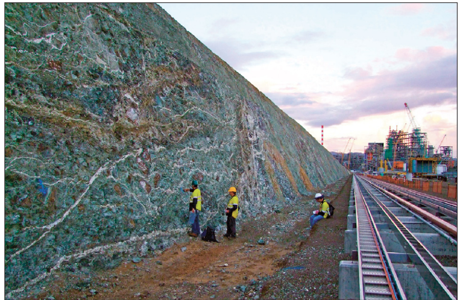
Figure 2. Field view along part of BMS cross section (located in Fig. 1B), illustrating exceptional size and freshness of outcrops recently opened in serpentine sole of Koniambo massif.
