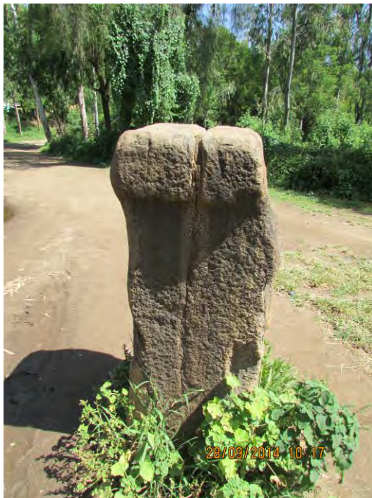
Fig. 5.62 Pillar 5, facing north. Note, the crack can be seen at the center of the pillar running from top to bottom (Photo: Hiluf Berhe, 28/09/2014).
