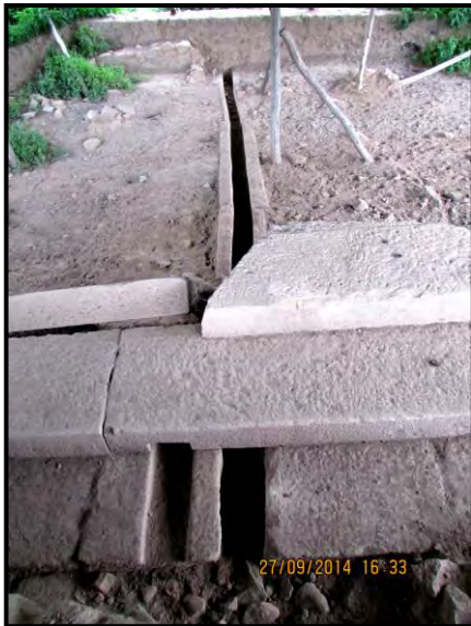
Fig. 4.19 Steps and drainage in area S at Ta'aka Maryam re-exposed by EEF/AkU in 2014 (view from north) (photo: Hiluf Berhe, 27/09/2014).
