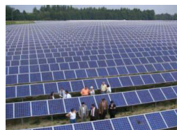
Figure 22: Megawatt scale PV power plant (INES, 2007, p. 10)
