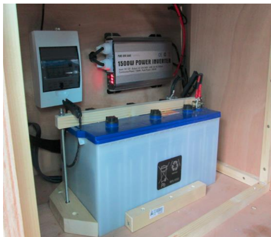
Figure 41 Power supply for the set-up (battery and inverter)
