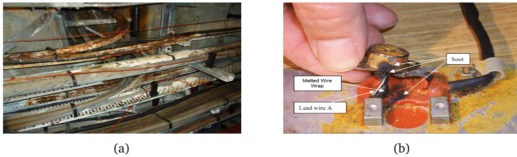
Figure 1.8 Samples of damaged cables: (a) due to moisture and humidity, (b) aircraft cable damage due to heating.
