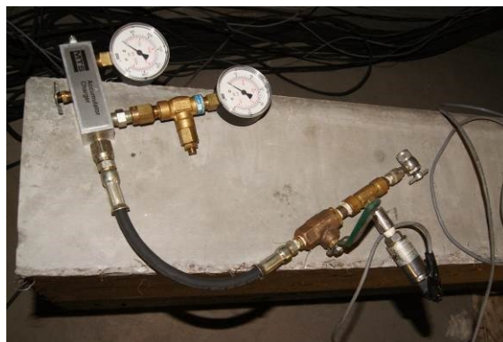
Valve de chargement d'azote (Subdivision 2)
