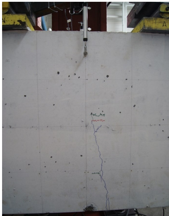
Figure B-28 : Faciès de fissuration
