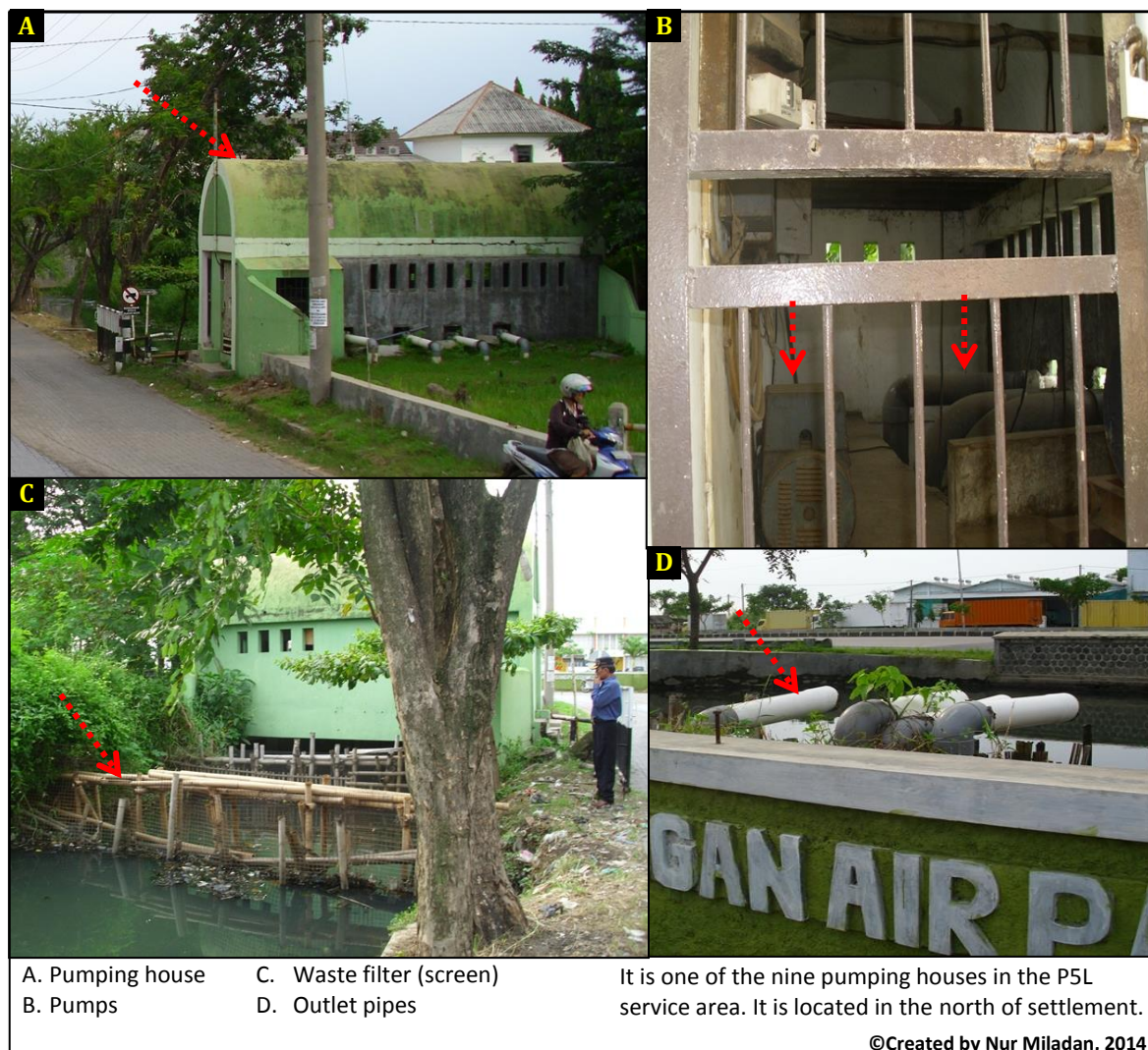
Figure 125. The pump system of P5L association
