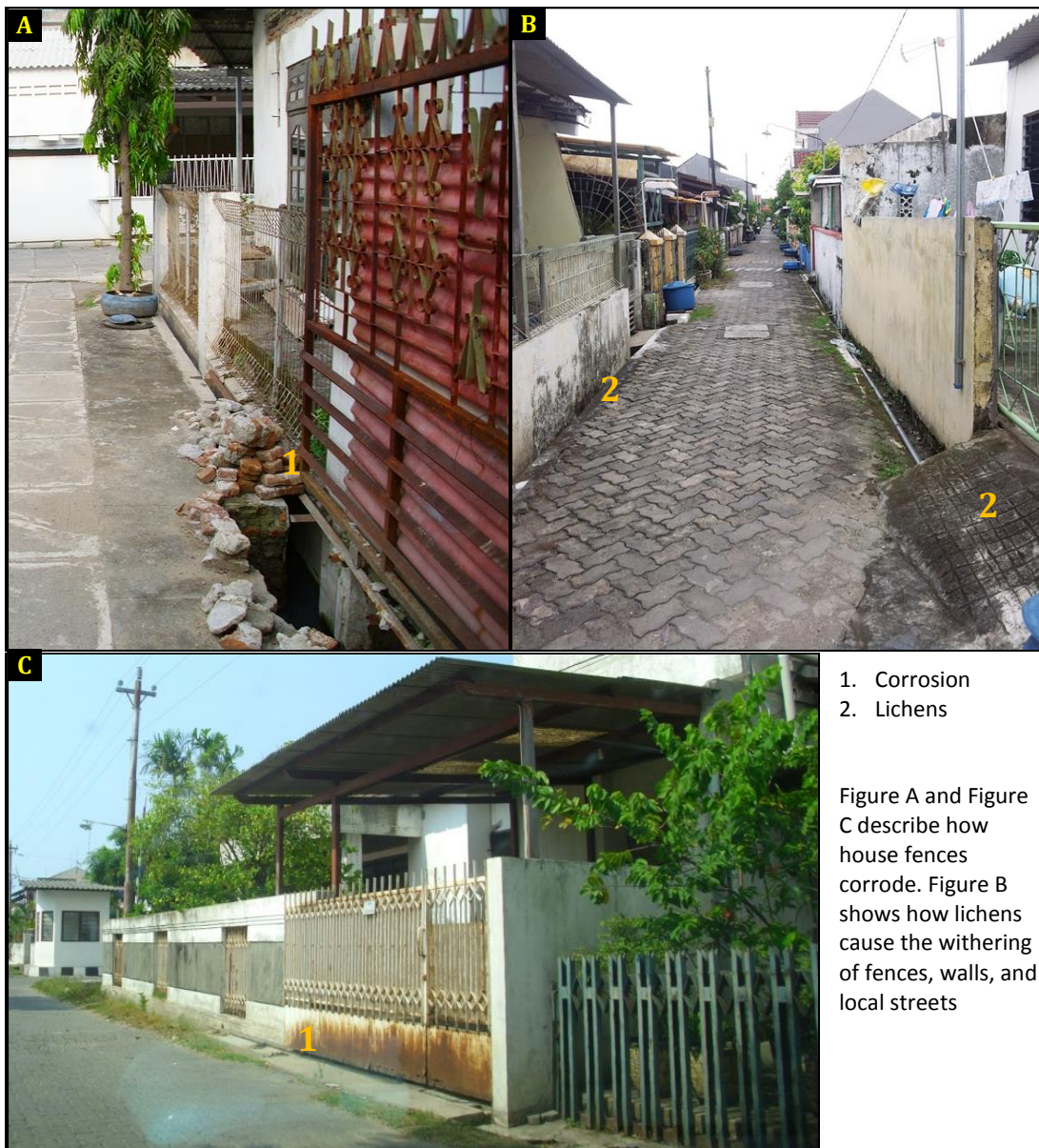
Figure 103. Lichens and corrosion on houses
