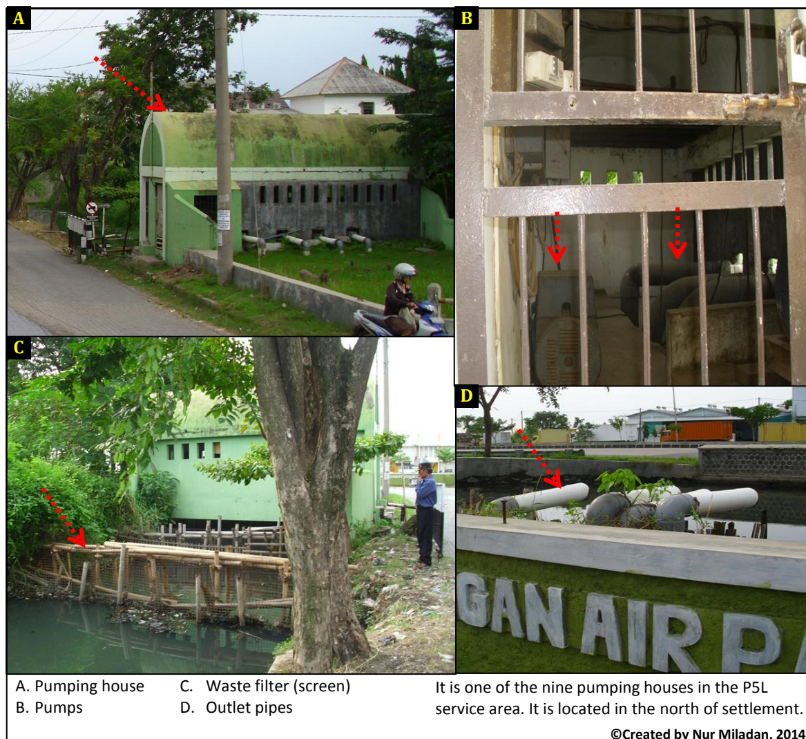
Figure 125. The pump system of P5L association
