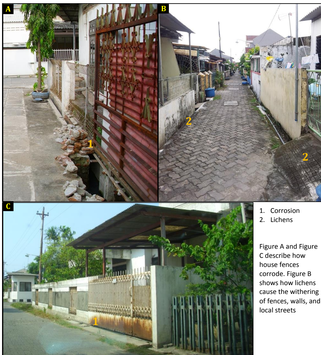
Figure 103. Lichens and corrosion on houses
