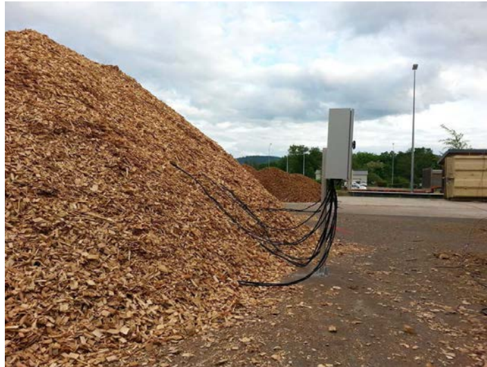
Figure 4.36: Security box for coaxial cables.
