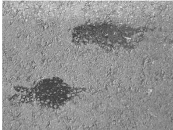
Figure 2-17 Damage to asphalt observed from the use of vegetable based ARA on new pavement
