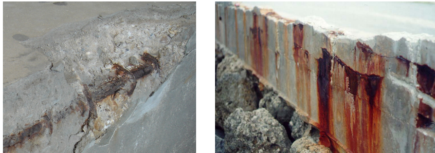
Figure 1: Example of degradations in a reinforced concrete medium
