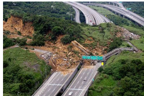
Figure 1.6 – Landslide burying a six-lane motorway in Taiwan.
