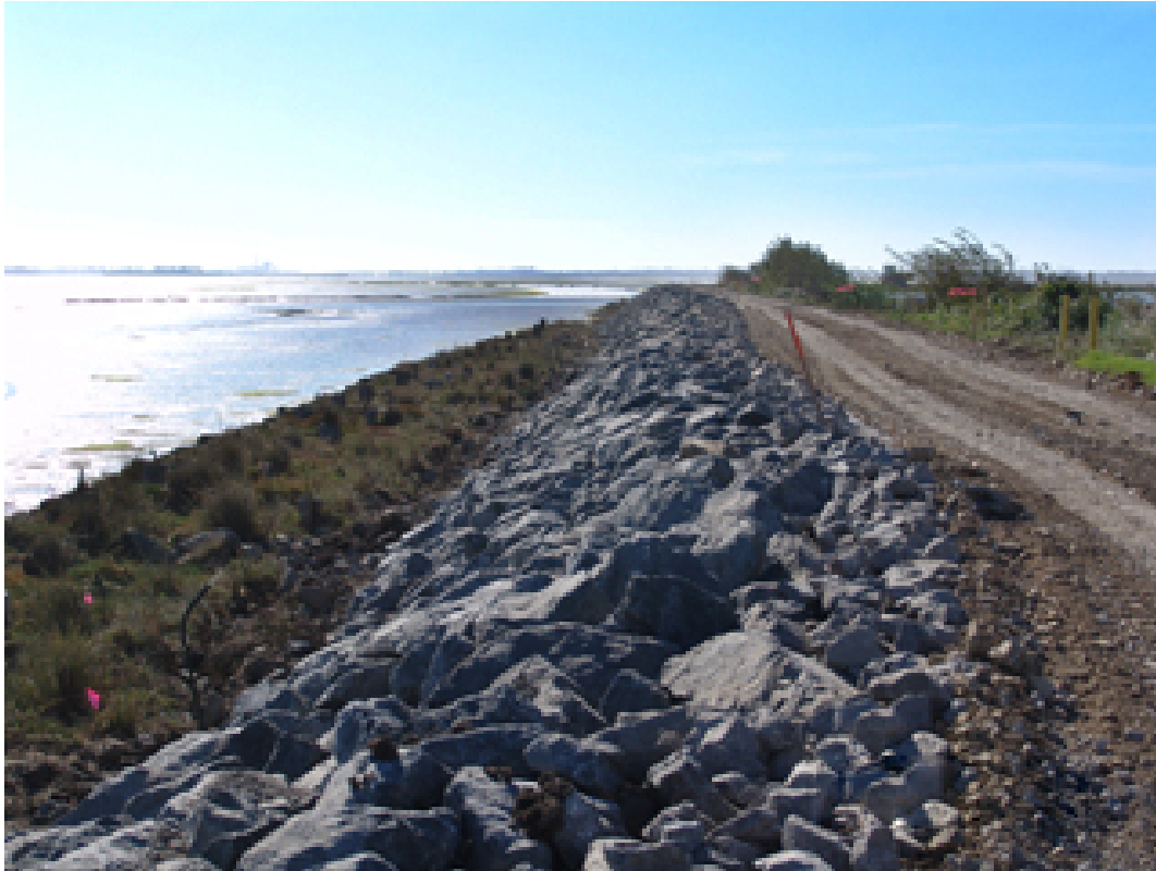
Figure 1.5 Coastal levees protecting Arcata waste water ponds from Humboldt Bay, California. Without levees protecting them, the waste water ponds flooded frequently. [California Gov, 2016]
