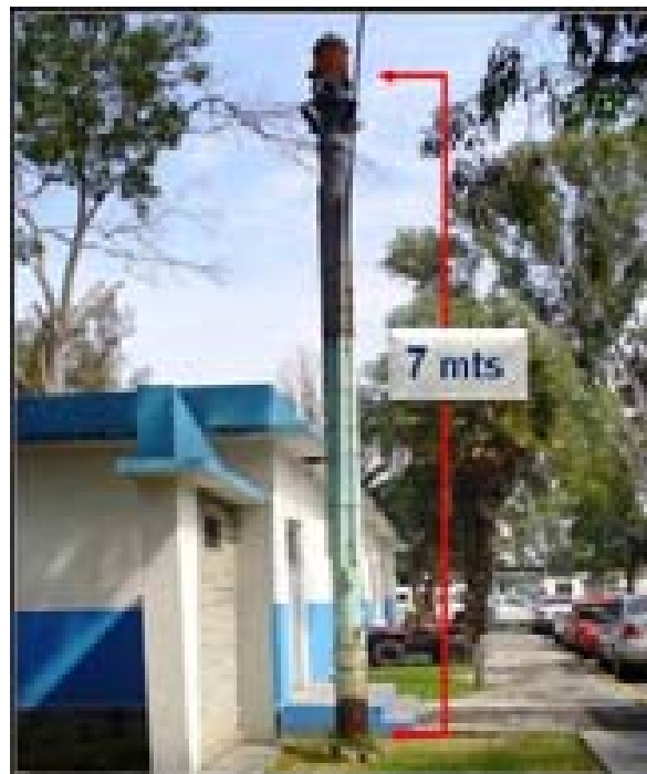
Figure 3.8 Water pump showing the soil subsidence. [Luege, 2012]
