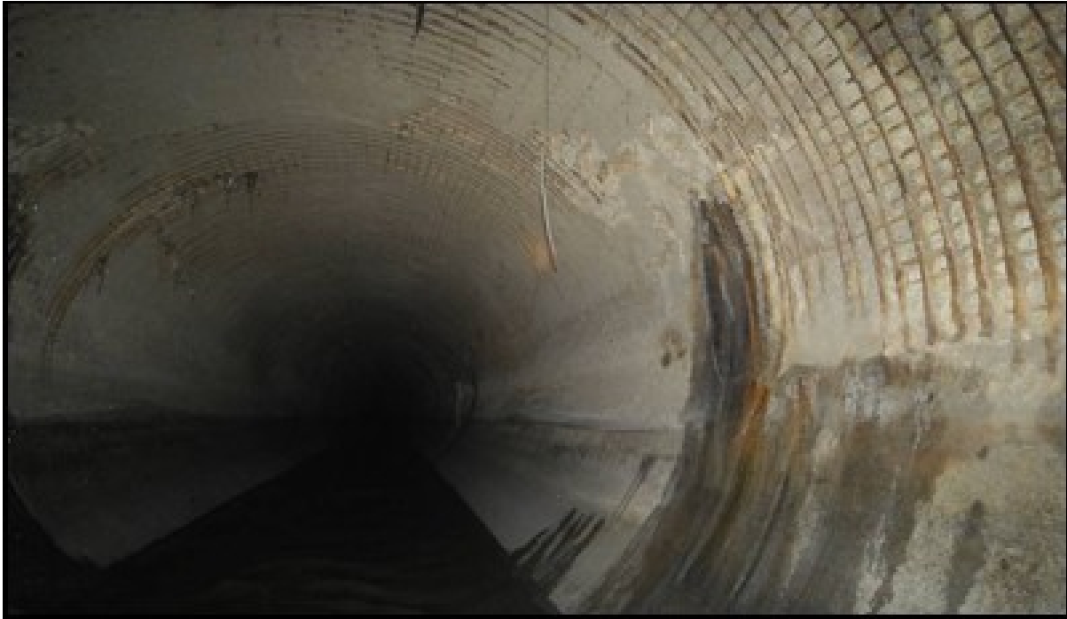
Figure 3.9 Internal deterioration of the Central Drain. [Luege, 2012]
