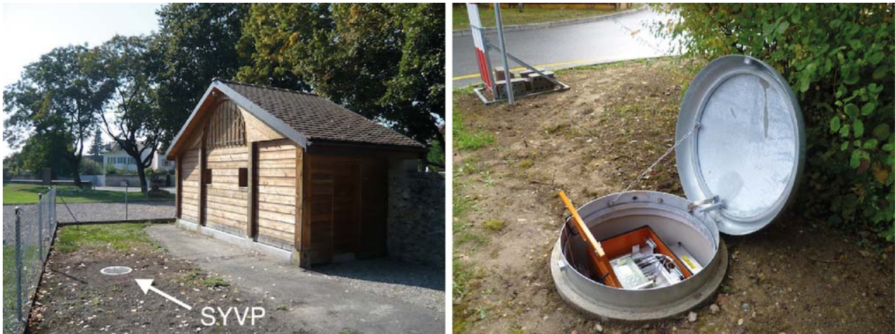
Figure 2. Alternative housing of the stations installed within the SSMNet renewal project. Left: small vault containing the sensor only and hut hosting the cabinet with the digitizer and communication instruments (station SYVP). Right: large vault containing the whole station (station SEPFL). The color version of this figure is available only in the electronic edition.
