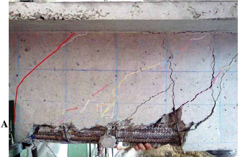
Figure A. 15. Cracking pattern Sample 3.
