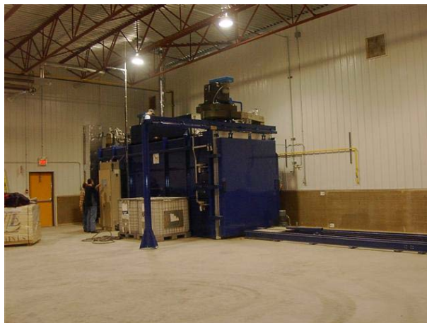
Figure 28: Four Perdure® 12 m 3 [PCI Industries Inc.]
