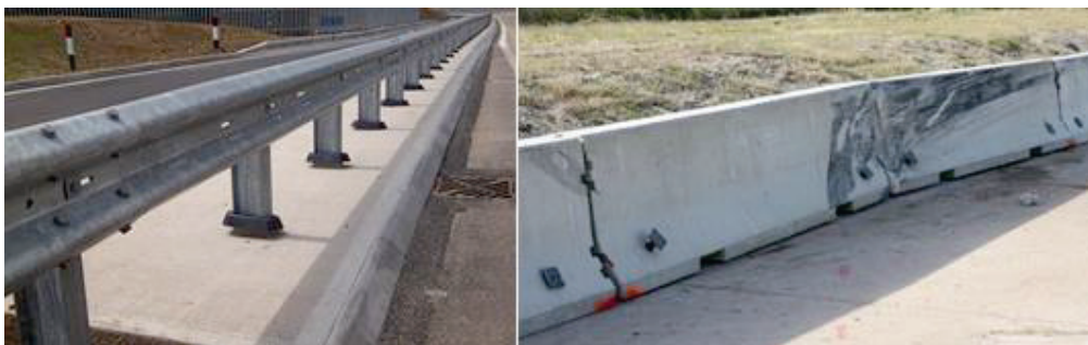
Figure 1- 5 Soft steel permanent VRS and rigid concrete temporary VRS (safety barrier)
