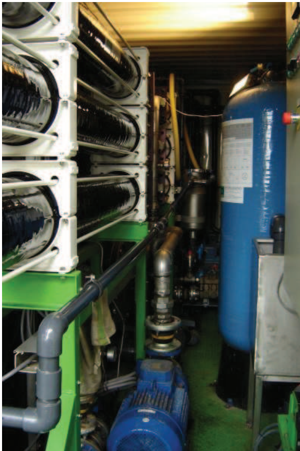
(b) Containerizable reverse osmosis plant. Source: http://www.lenntech.com
