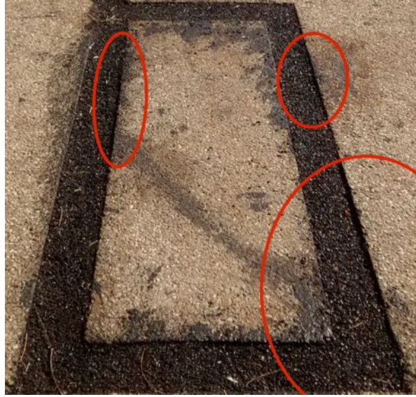
Figure 7.26: Deteriorated areas (red circles) on coil L_5 .
