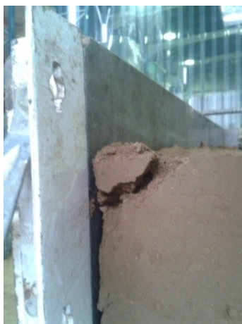
Figure 1.12: Tear of a corner while removing the formwork.
