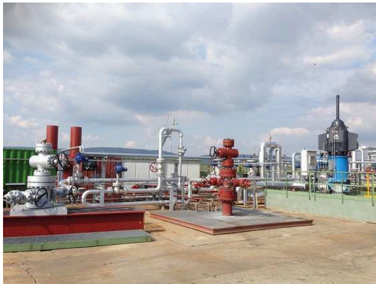
Figure A.1. Surface equipment of the EGS in Soultz-sous-Forêts (wellheads)
