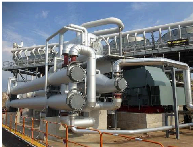
Figure A. 3 Surface equipment of the EGS in Soultz-sous-Forêts (ORC equipment)
