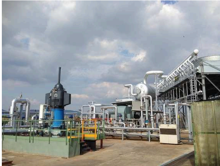
Figure A.2 Surface equipment of the EGS in Soultz-sous-Forêts (panoramic view)
