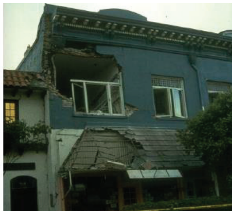
Santa Crus, Loma Prieta (1989)
