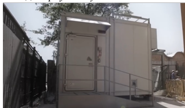
(c) SF's micro DC final installation
