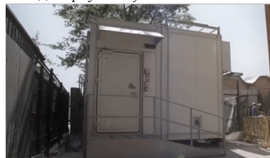
(c) SF's micro DC final installation
