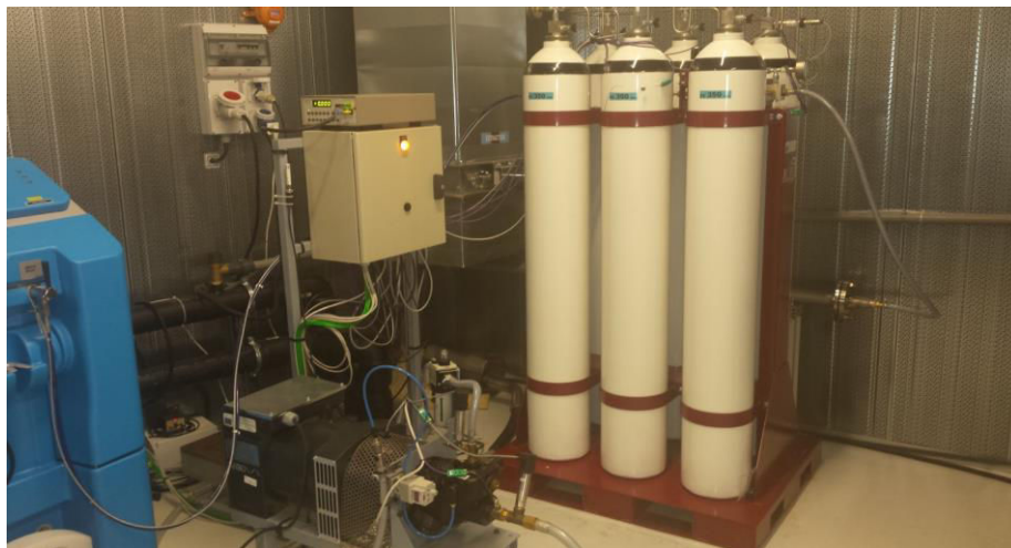
Figure 57 – Storage vessel side view
