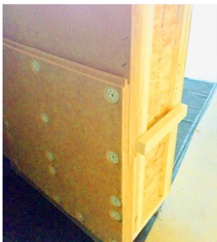
Figure 154. Top. BIM model including carpentry data. Bottom. Wall curvature second solution by full-scale prototyping. A 2x10 mm OSB sheathing replaces 18 mm sheathing for achieving a smoother bending and avoid breaking. Top image courtesy of Dform architecture. Bottom image J.M.
