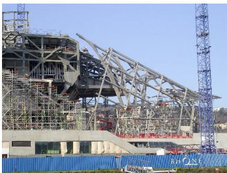
Figure 36. Bearing and façade structures for the Confluences Museum at Lyon-France, by Coop Himmelblau. Photo 2012, O. GAMEZ.
