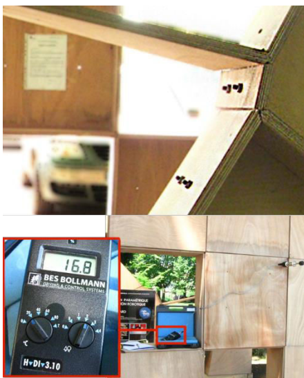
Figure 187. Top: Visual inspection and gap measurement showed no dimensional changes in items exposed to open-weather conditions. Bottom: Moisture measurement on rain-exposed cells.
