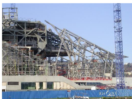
Figure 36. Bearing and façade structures for the Confluences Museum at Lyon-France, by Coop Himmelblau. Photo 2012, O. GAMEZ.
