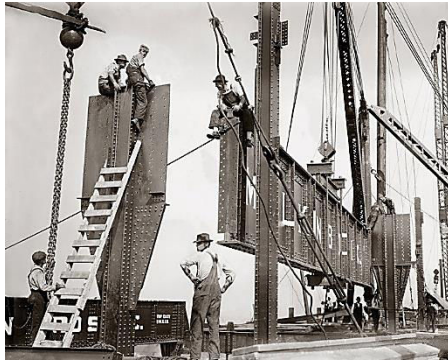
Figure 6. Steel workers mounting a pre-assembled girder for the Consolidated Gas Company Building. N.Y 1913. Source: etsy.com
