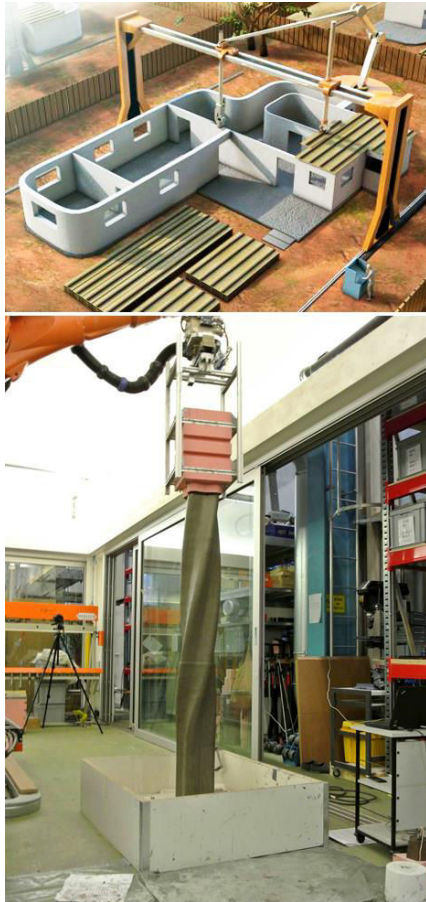
Figure 105. Top. Contour Crafting technology as conceived by B. Khoshnevis (2013). The extrusion head, driven by a gantry robot, pours layers of mortar as it displaces along a construction path. On: dailymail.co.uk/sciencetech . Bottom. Smart Dynamic Casting method (Lloret et al., 2015) gradually pours fine-aggregate low-retraction concrete as the extrusion pre-shaped nozzle also gradually revolves on its own axis. The method allows for casting concrete columns with different shaft morphologies without the help of any fixed formwork. On: http://gramaziokohler.arch.ethz.ch/web/e/forschung/223.html
